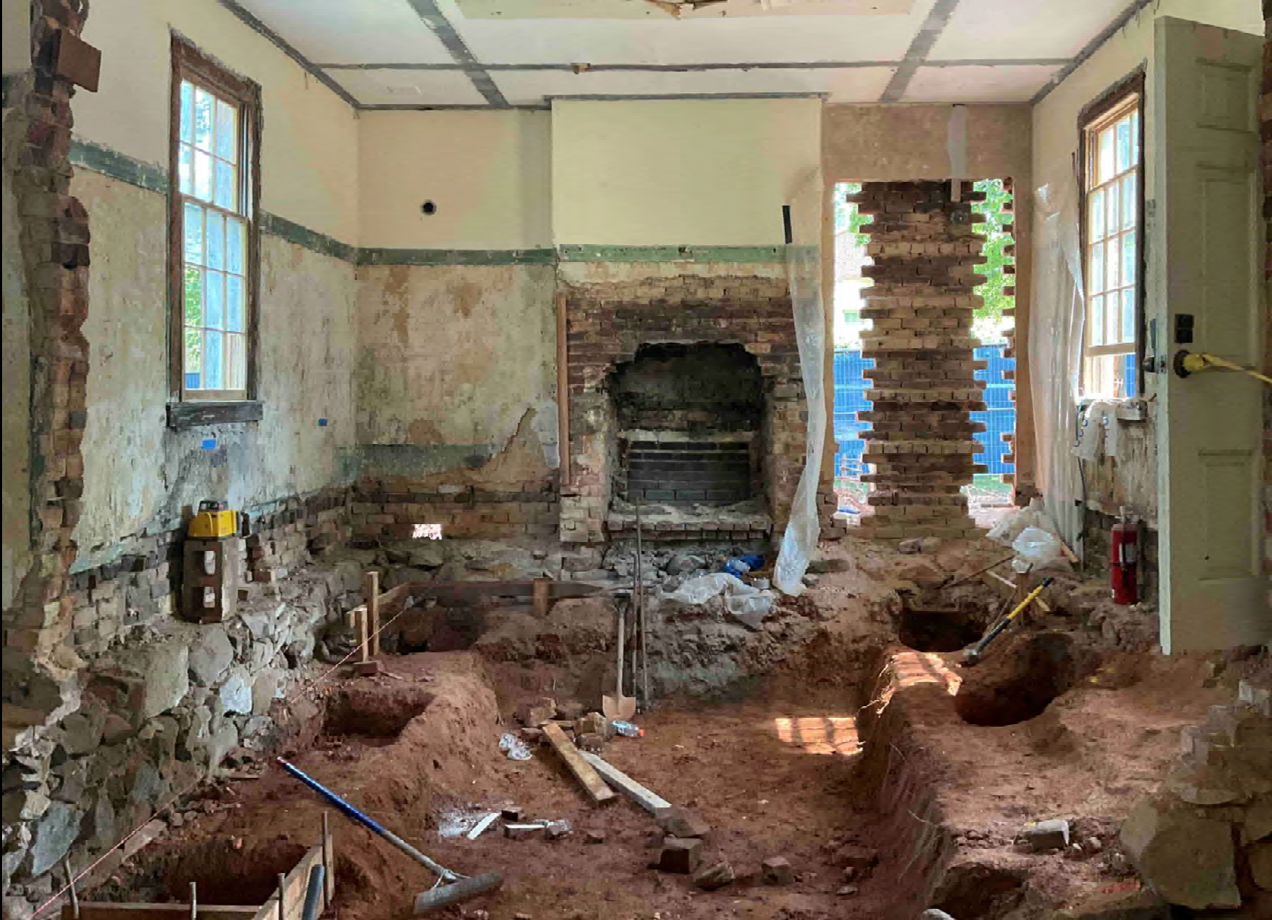
Images of the north elevation and interior during demolition. Floors were removed due to termite damage. New openings were created in the existing brick walls with great care. Fireplaces were opened and restored.
