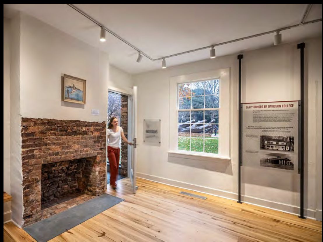
Reclaimed bricks from demolition were used to repair and stabilize the new openings and uncovered original fireboxes.
