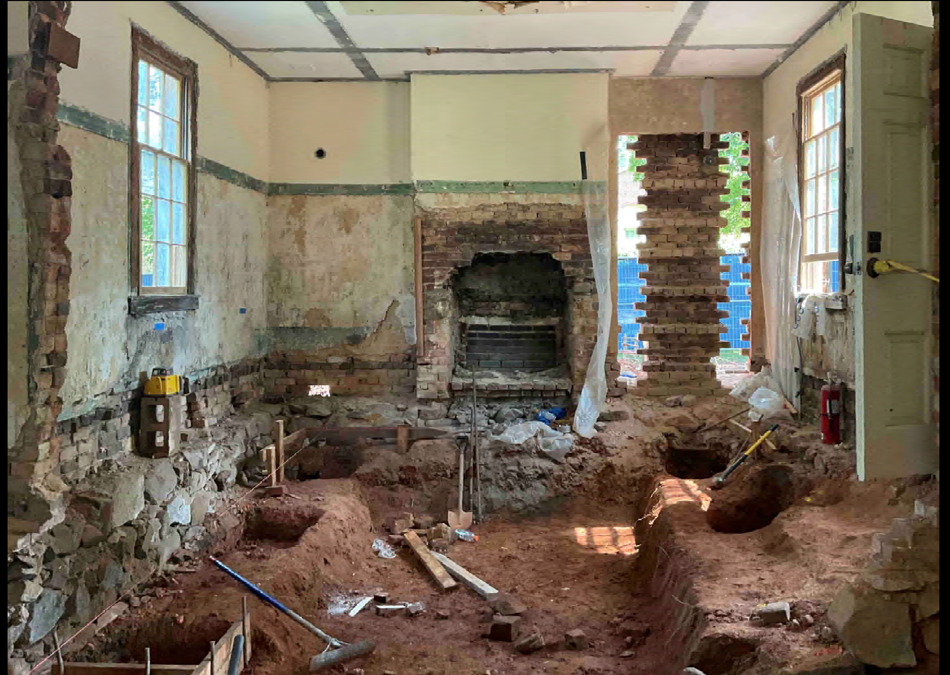
Images of the north elevation and interior during demolition. Floors were removed due to termite damage. New openings were created in the existing brick walls with great care. Fireplaces were opened and restored.
